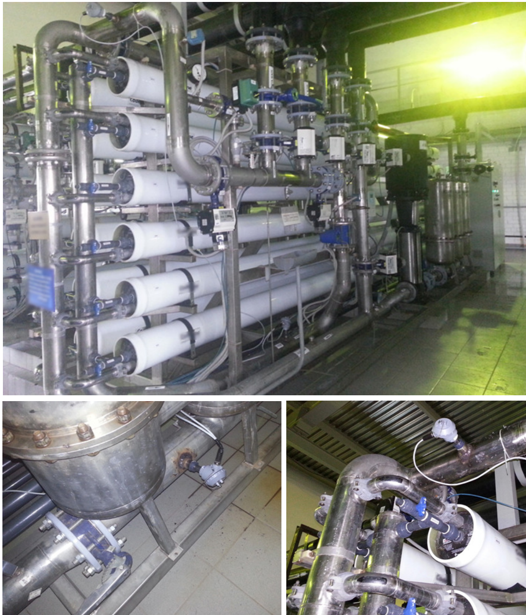
Figure 3: Overview of RO system (on the top), ALVIM Sensor installed before RO (on the bottom, left), ALVIM Sensor installed in the concentrate line (on the bottom, right).
